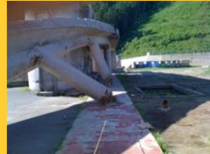
Ookawa elementary school broken by Tsunami
